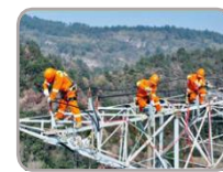
Direct Current De-Icing: Operation is complex energy consumption is high.
