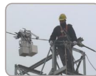
Robotic Mechanical De-Icing: It is difficult and highly dangerous to install robots on iron towers after they have iced up.
